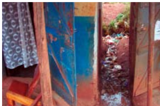
Poor drainage. Photo: © Kampala city council
